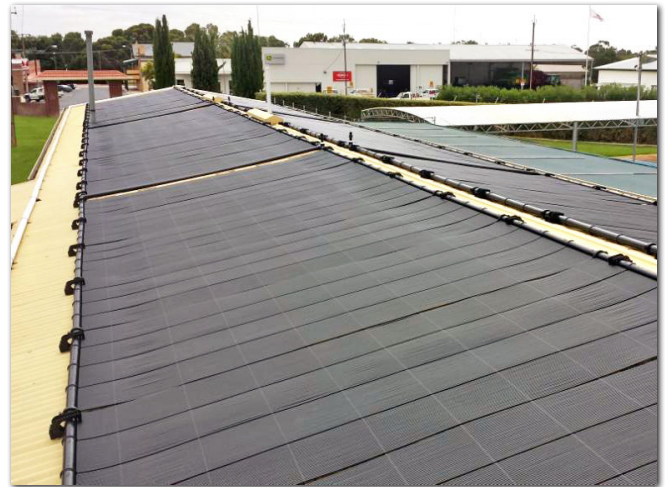
New Heliocol solar pool heating system.
